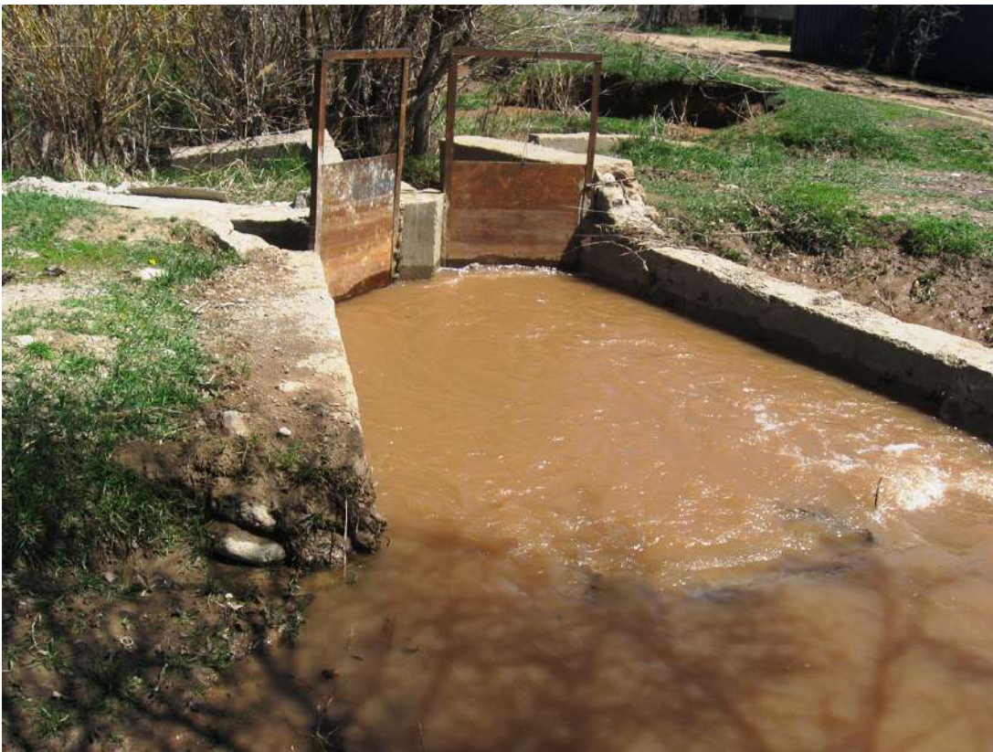
Picture 4. Distribution structure which is subject to rehabilitation, 02 May, 2015
